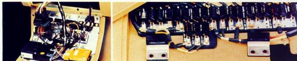
Electrical distribution center.
