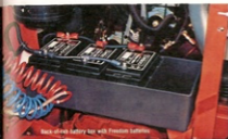
Back view battery box with Freedom batteries
